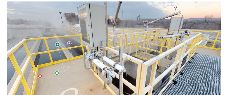
Chlorine Contact Basins (CCBs) at the Lower Meramec Wastewater Treatment Facility, shown here at a facility owned by the Metropolitan St. Louis Sewer District, were a part of Jearls’ earliest WWTF design experiences. After the flow to the treatment facility has been treated through primary and secondary processes, it is disinfected at the CCBs by means of chlorination and de-chlorination.
